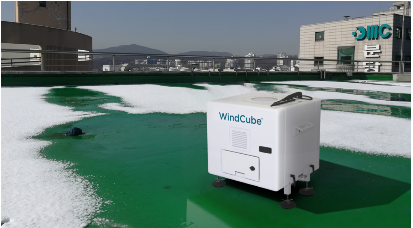
Figure 13: Urban WindCube deployment — WindCube v2 deployment at VisionPlus Korea.
