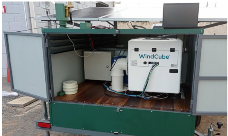
Figure 17: WindCube integrated in a trailer with a cooling system attached to the lidar — Photo courtesy of Hobeco.
